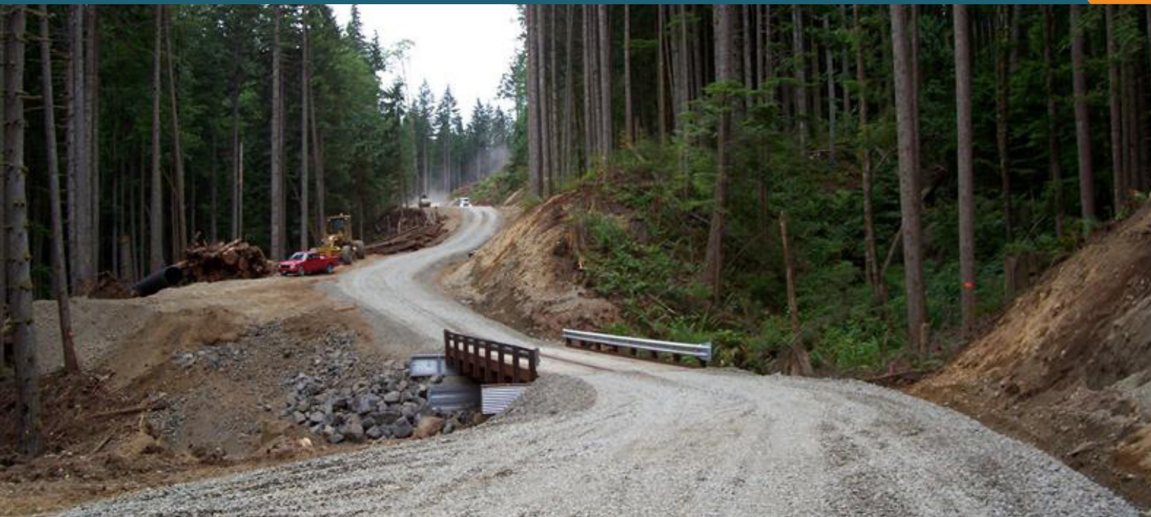
A newly constructed forest road, built as part of the Soderman Slope Timber Sale in eastern King County. Credit: Washington State Department of Natural Resources
