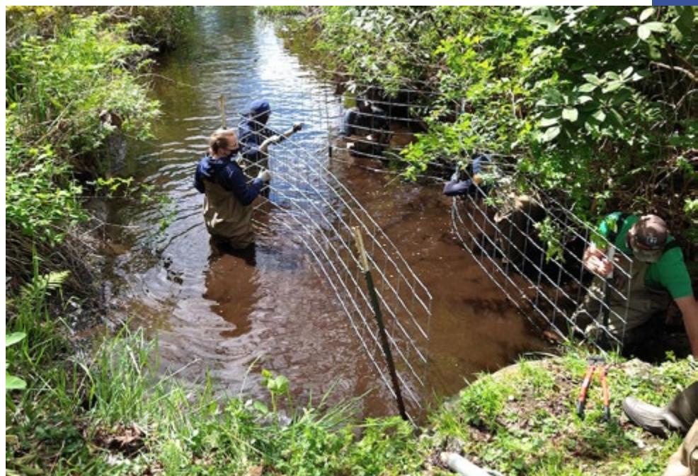
Exclusion devices, like the one seen here on Stitch Creek in Lake Stevens, being installed in front of a road culvert, can prevent problems caused by beavers. Photo: Courtesy Snohomish Conservation District
