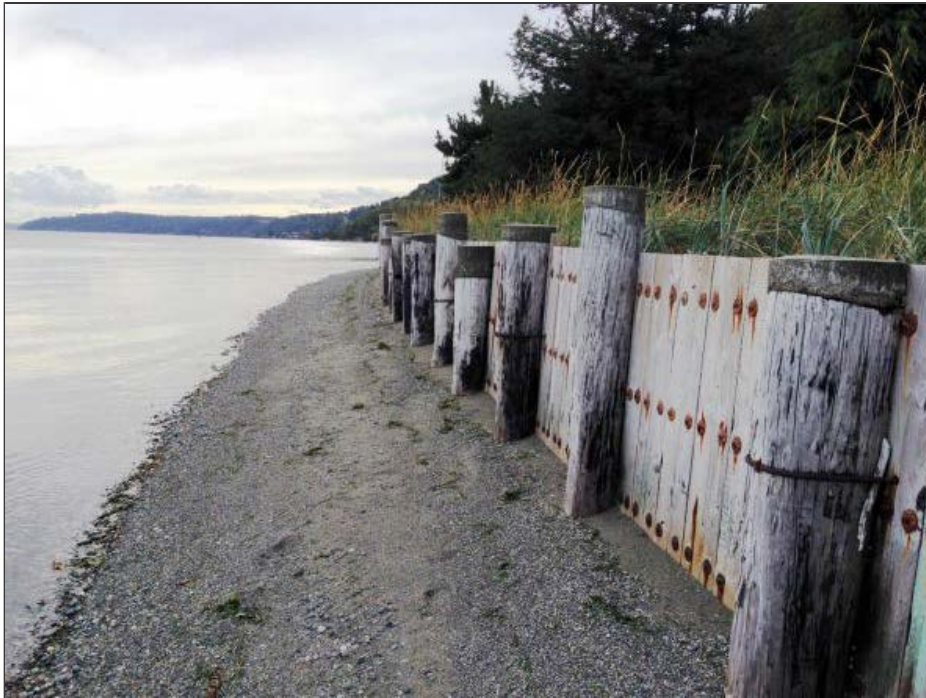
The neighbor's bulkhead confines the beach to a narrow strip of gravel, similar to Pat Collier's beach before bulkhead removal. Every shoreline property is different, and this site offers a greater challenge because the house is closer to the shore. Photo: Christopher Dunagan/PSI
